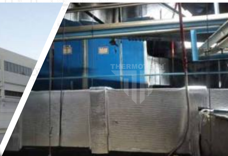
PROJECT NAME : UNILEVER SKIN ZARA APPLICATION PRODUCTS : DUCT INSULATION LOCATION : CIKARANG
