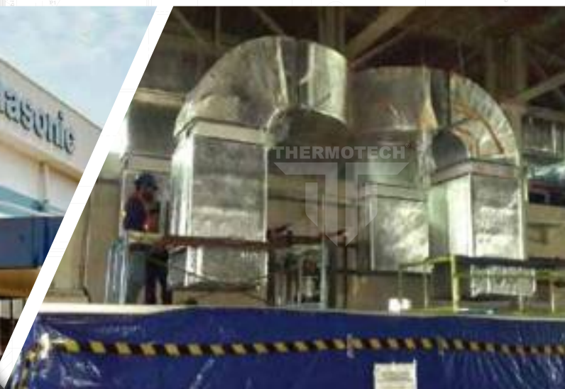
PROJECT NAME : PANASONIC HEALTH CARE APPLICATION PRODUCTS : DUCT INSULATION LOCATION : KAWASAN INDUSTRI MM2100
