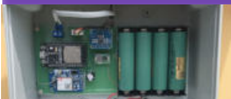
Sensors for battery power measurement
